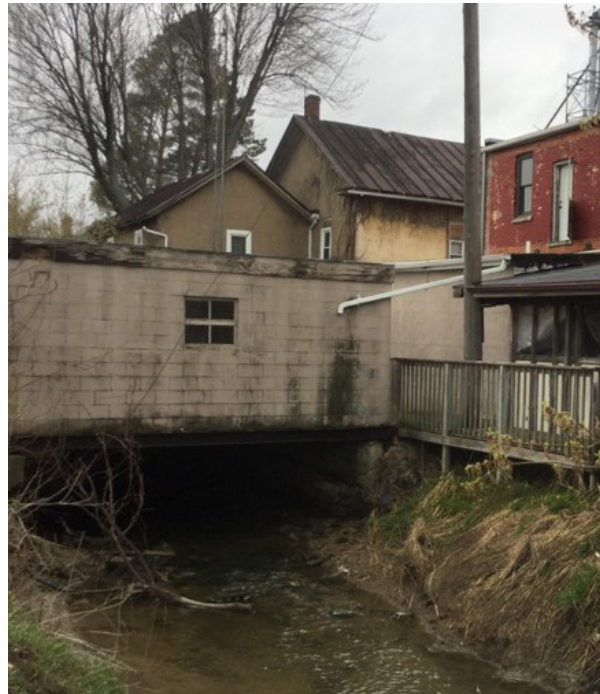
Structure built over a drain
