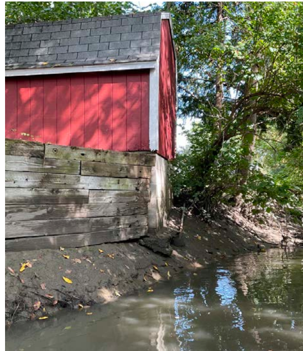
Shed built on drain easement
